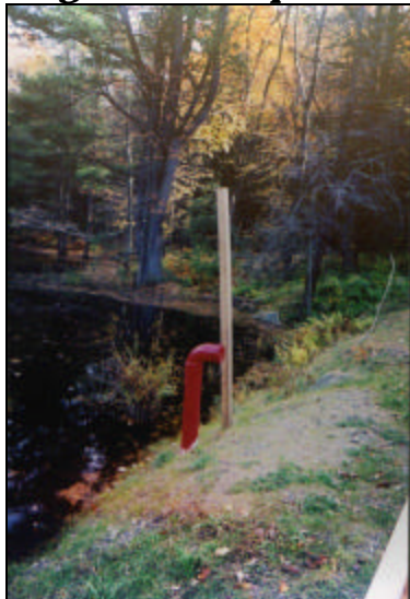
Dry Hydrants help fight fires in rural settings
